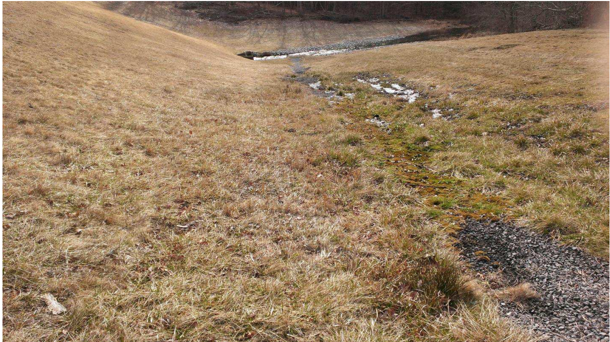
Seepage/wet area on west side of embankment
